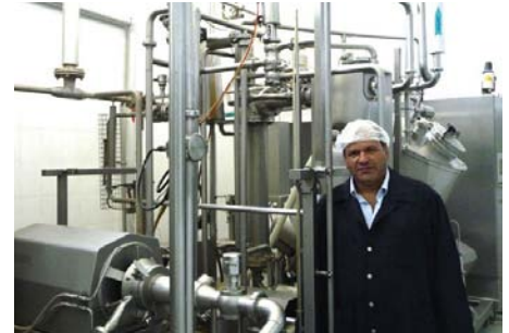
Technical Manager Hosny Ragheb in front of the first UHT, delivered in 2003: "The system - in operation for 8 years - is still in good condition."
